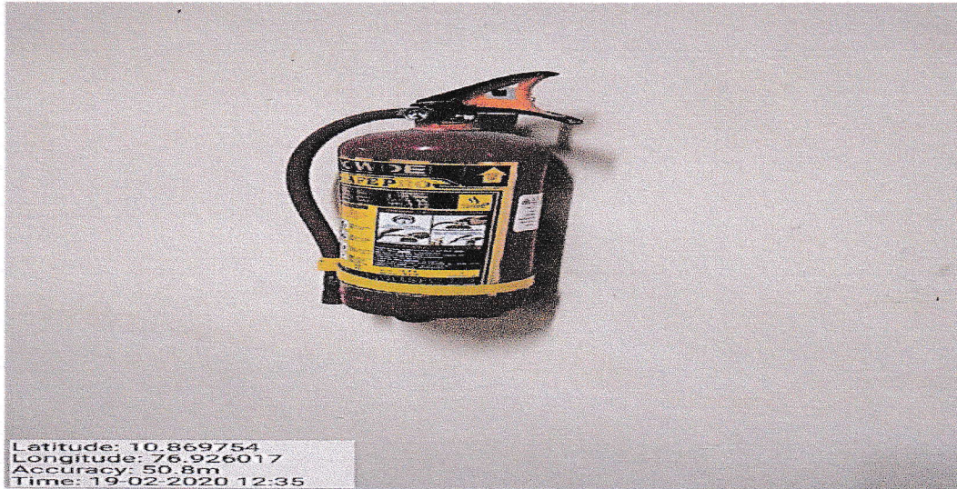
Fire Extinguisher at each floor
